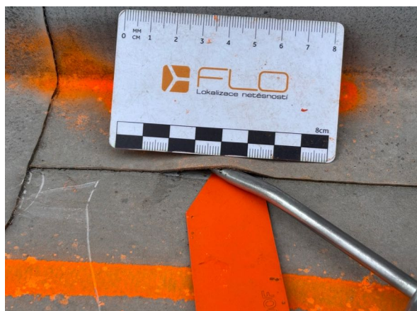
Obr. 25 Defekt B1 detail
