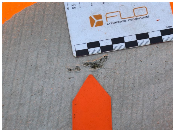
Obr. 8 Defekt A2 detail
