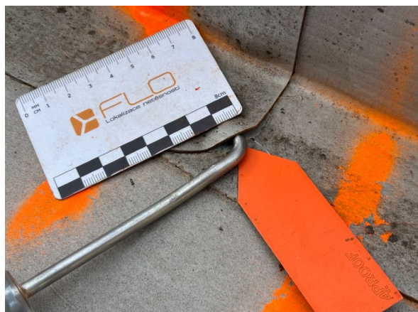
Obr. 27 Defekt B3 detail
