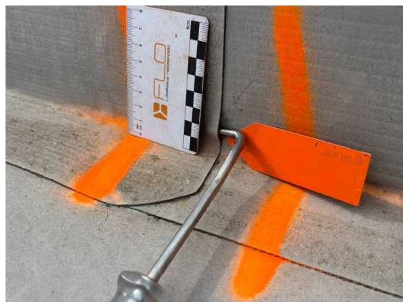
Obr. 28 Defekt B4 detail
