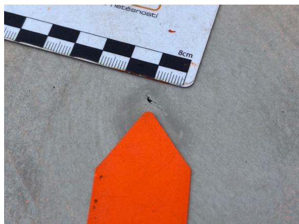
Obr. 6 Defekt A1 detail
