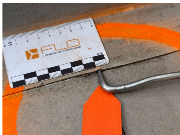
Obr. 30 Defekt C1 detail
