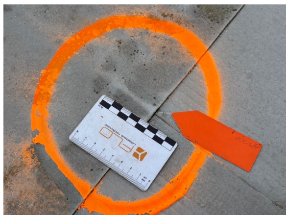
Obr. 14 Defekt C1 detail
