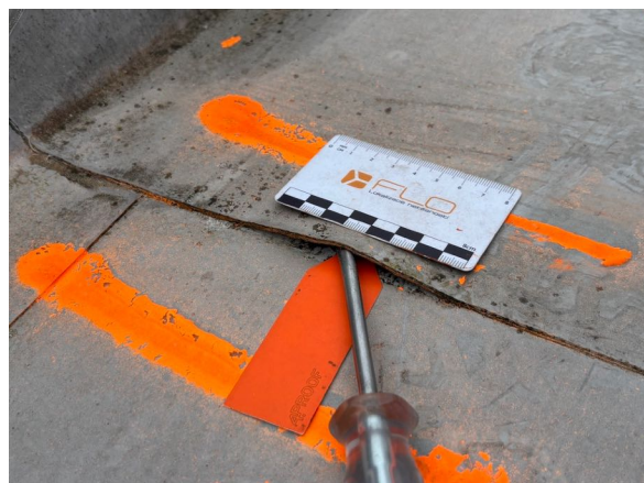
Obr. 12 Defekt B8 detail
