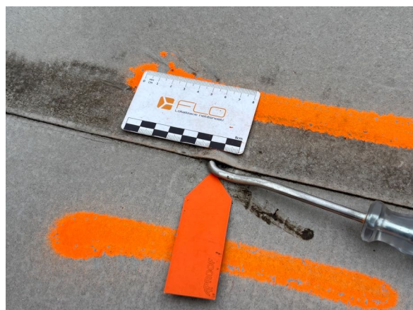
Obr. 26 Defekt B2 detail
